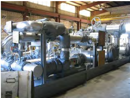
Intercooler Water Circ. Package Customer: GE/Basin Electric
