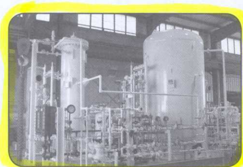
IFS Fuel Gas Conditioning Package for Mexico's Pemex Offshore project
