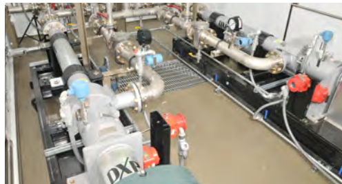
Water Transfer Skid
