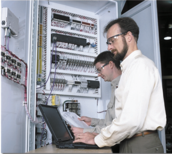
IFS electrical and mechanical engineers are experts in automation and controls design. Each project requires careful controls engineering to guarantee proper field operation and to ensure that the system will perform to specifications.
