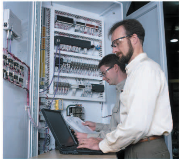
Downloading pre-tested programs into the PLC for complete package testing.
